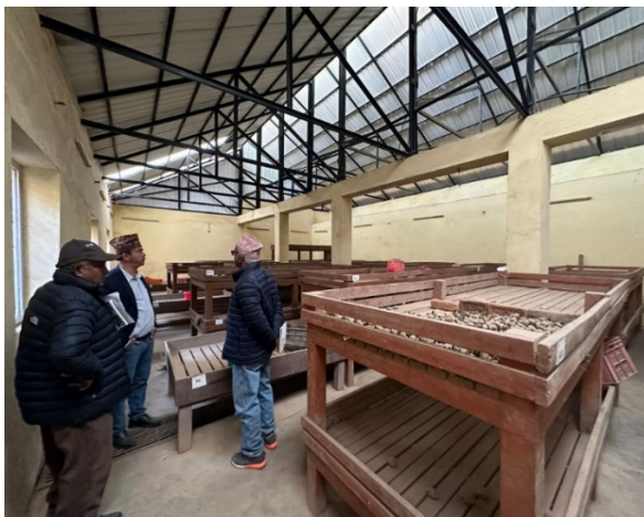
Rusting House Inspection.
